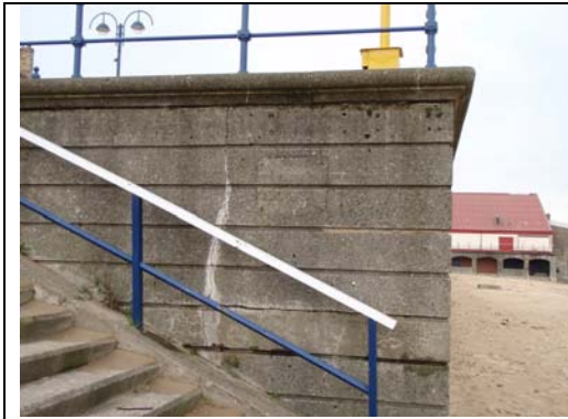
Settlement/movement of seawall (Asset Ref No 1221C901C0602C04)
