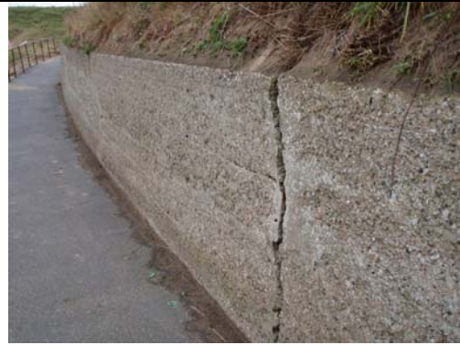
Crack in concrete wall below coastal slope (Asset Ref No 12221C901C0702C02)
