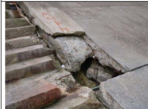
Failure of previous repair exposing reinforcement and infill material (Asset Ref No 1221C901C0602C01)
