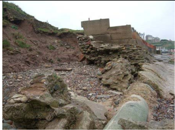
Total collapse of part of concrete defences and failure of unprotected cliffs (Asset Ref No. 1221C901C0704C05)
