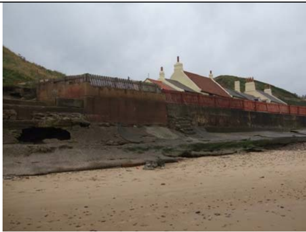
Property at risk behind eroded concrete defences (Asset Ref No. 1221C901C0704C05)
