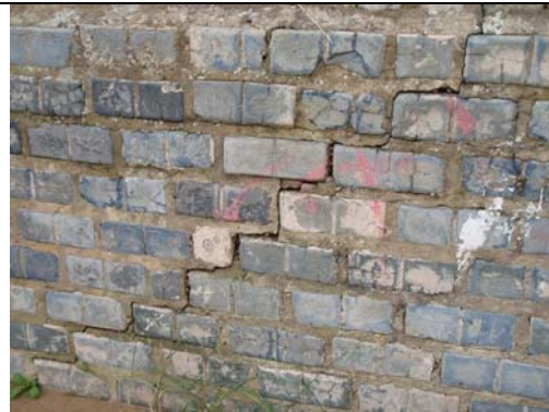
Settlement crack in masonry wall (Asset Ref No 12221C901C0702C01)
