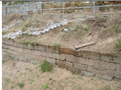
Missing masonry blocks with erosion and vegetation growth below (Asset Ref No 12221C901C0702C02)
