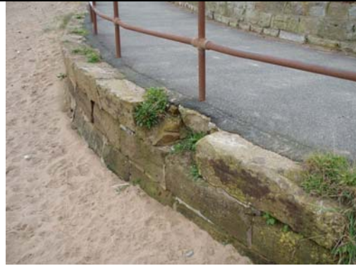
Missing masonry blocks and mortar with vegetation growth in gaps (Asset Ref No 12221C901C0702C02)
