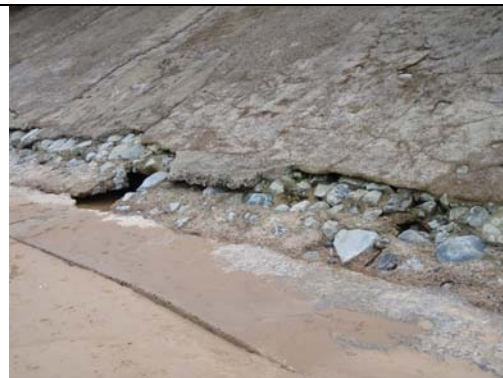
Erosion at toe exposing masonry and forming voids (Asset Ref No 1221C901C0602C01)
