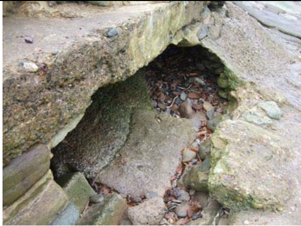
Undercutting and excavation of concrete defences (Asset Ref No. 1221C901C0704C05)
