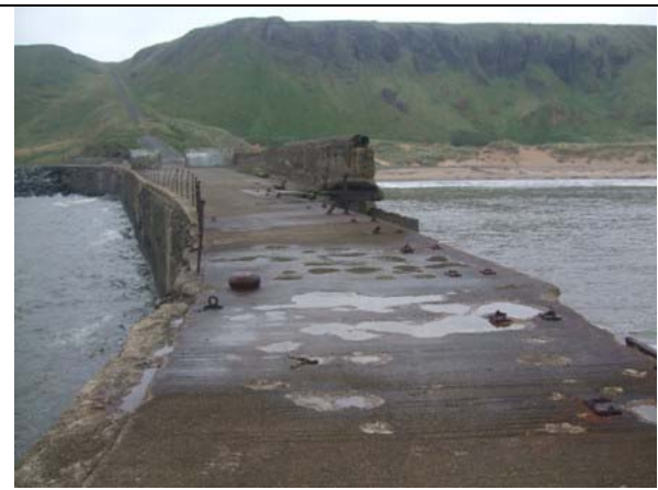
The jetty west of Skinninggrove (Asset Ref No. 1221D901D0201C02)
