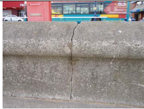
Crack propagating from construction joint (Asset Ref No 1221C901C0602C02)
